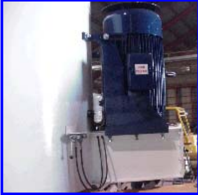
Bolts securing Motor Stand are outside Belt Tunnel
