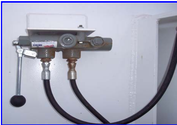
Grease Valve– splits between Top and Bottom Bearings
